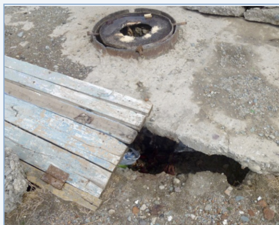
Figure 5. Typical open hole for biological waste.
